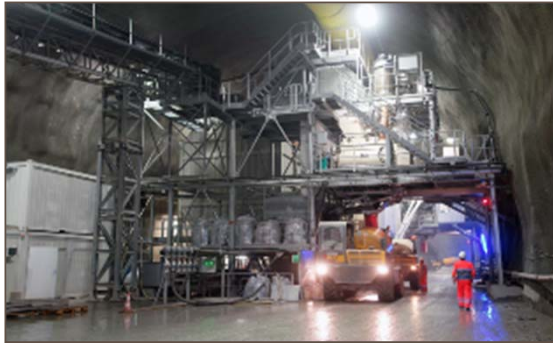
Tailor-made underground RMX plants (24h delivery)
